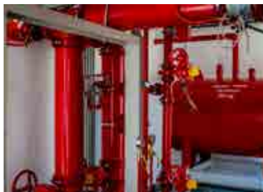
FPS / Fire Protection Solutions
